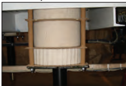
CT's (Bushing mounted internally)
