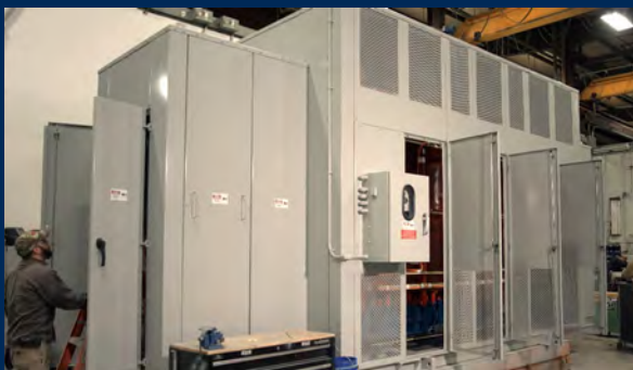
UNIClad transformer in Roanoke
